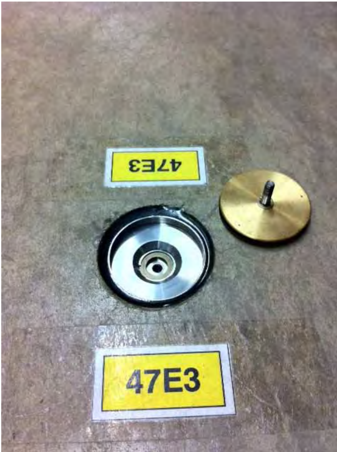
Figure 2.120: Floor target with cover removed.
