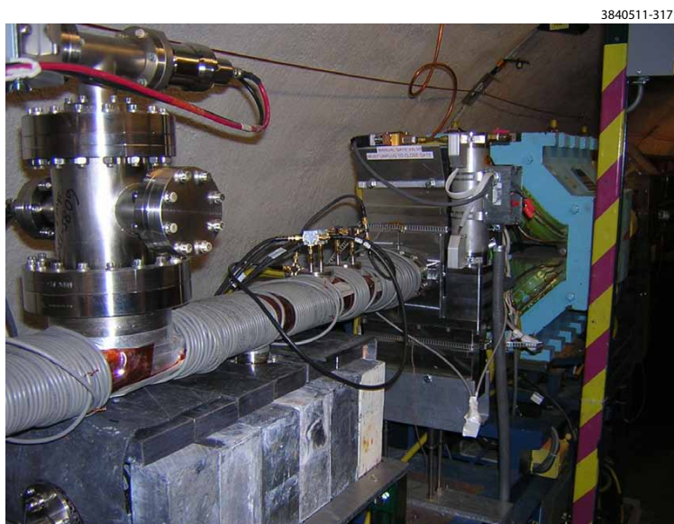
Figure 2.130: View of solenoid windings on a second typical arc vacuum chamber.
