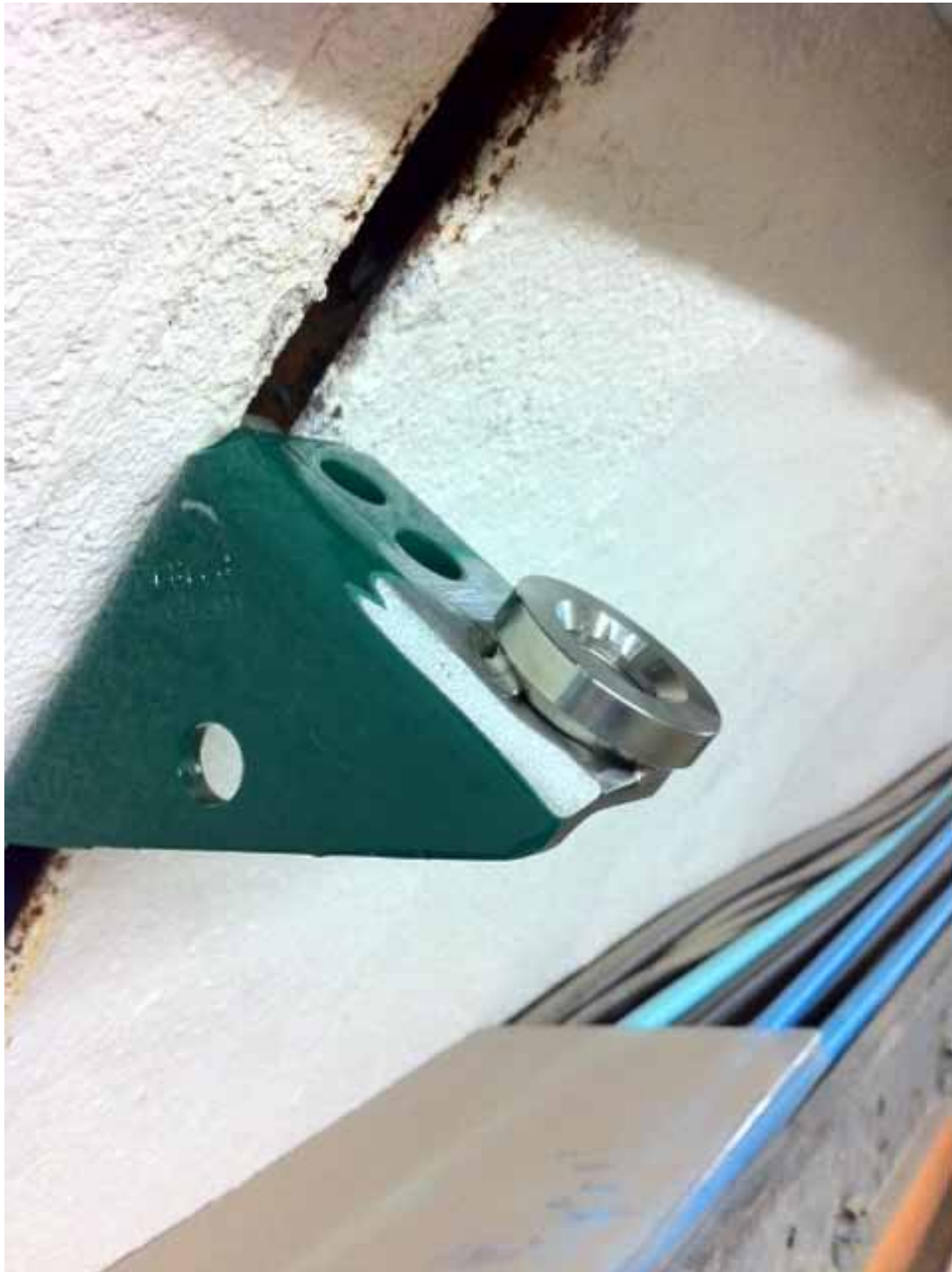
Figure 2.118: Wall Target attached to tunnel Uni-Strut.
