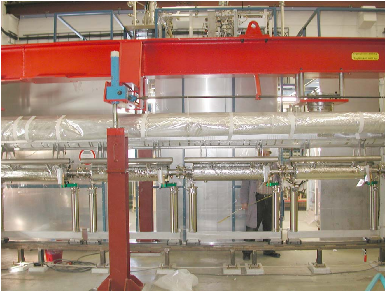
String in the assembly area
