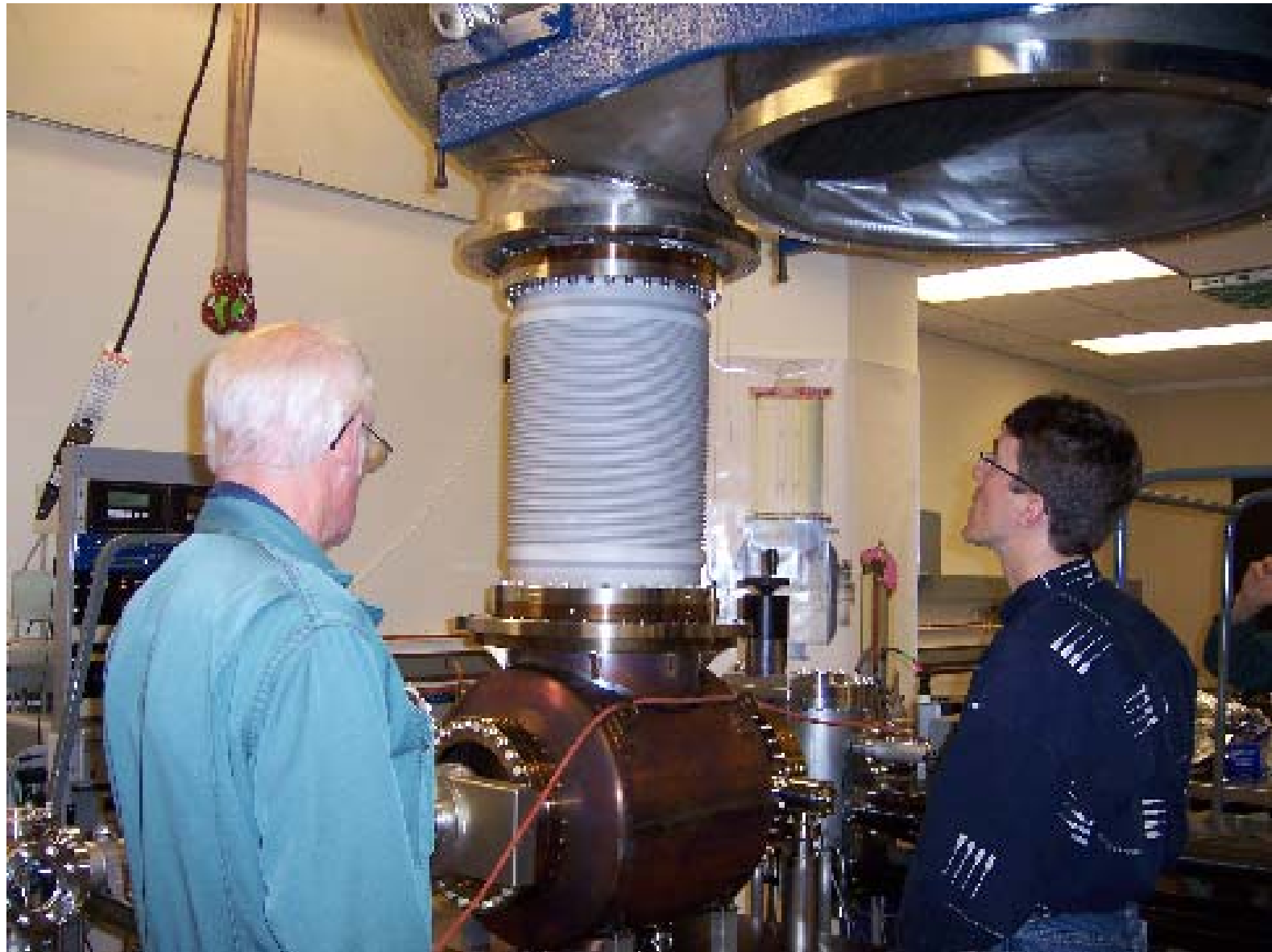
Installing the SF 6 tank over the large ceramic insulator of the electron gun
