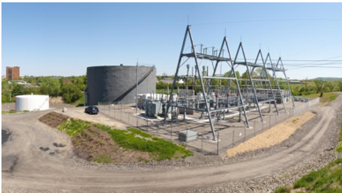
Figure 4.4.2: Maple Avenue substation.
