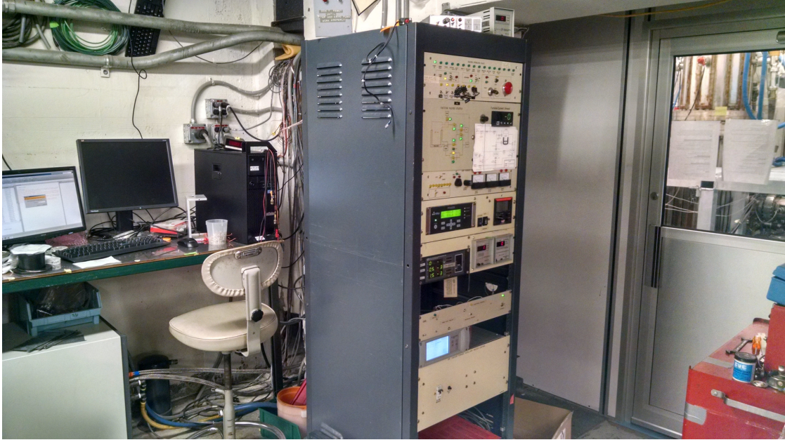
Figure 3.10: The control system for the Cornell coating furnace. Pumps and valves are operated from the central rack, which also hosts the power supply interlock. Once active, the furnace is controlled from the computer on the left. The furnace can be seen through the cleanroom door on the right.
