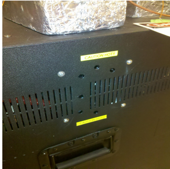
Figure 9: 6 1/4" drilled out holes to allow for better air flow from cooling fan
