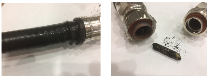
Figure 3.2.4: Damage to an internal cable connecting a single module to the power combiner in a 5 kW SSA which led to the failure of the associated power module.
